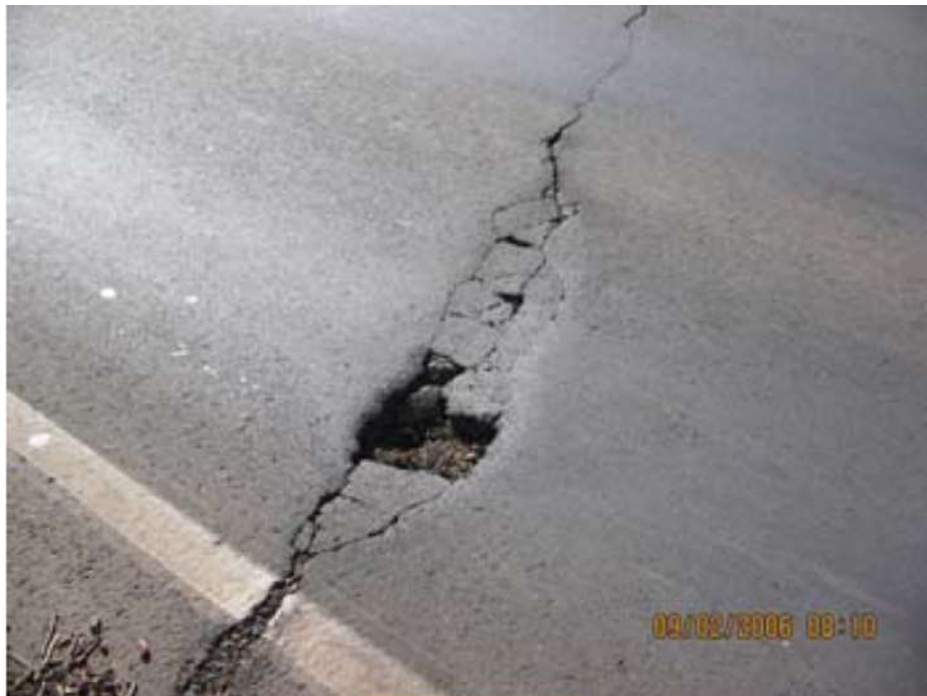
Figure 1: An example pothole (Photo NMDOT 2007)
