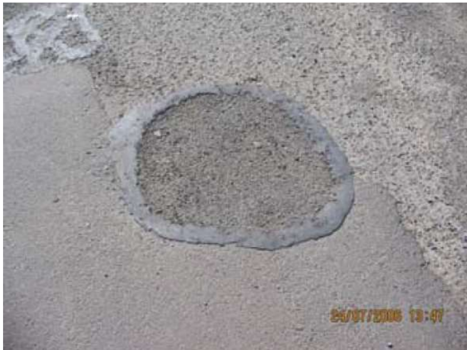
Figure 7: A properly repaired pothole. Note the sealing around the edges. (Photo NMDOT 2007)
