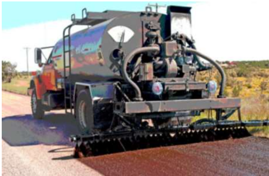
Figure 2: A fog seal operation is one type of preventive maintenance (Photo NMDOT 2007)
