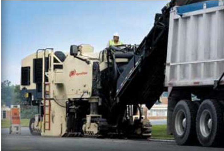
Figure 3: Milling must take place before the overlay of new asphalt pavement (Photo NMDOT 2007)
