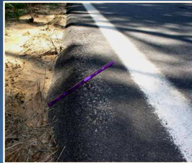
With Safety Edge
