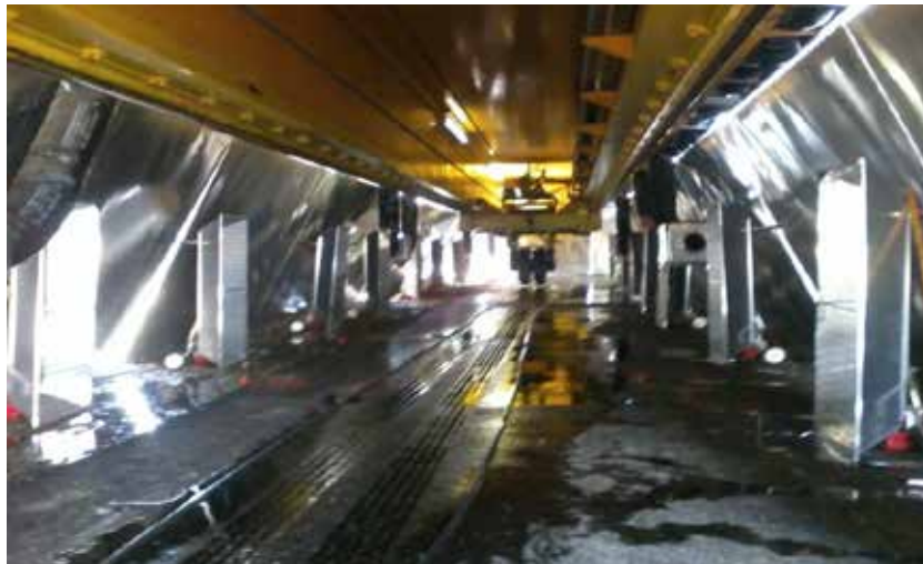
Figure 3.6 Heaters and shields under ATLAS.
