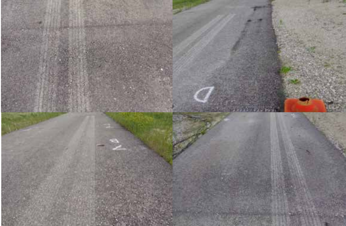
Figure 3.9 Several field sections showing possible mix uniformity issues.
