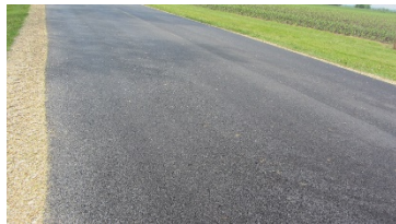
East Coral Road (Sections 1 and 2) after Overlay
