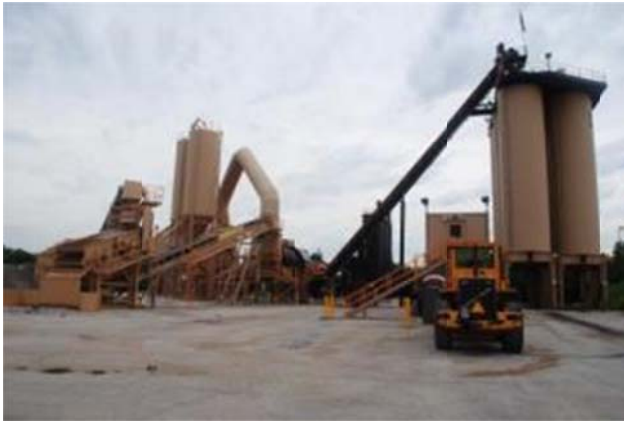
(a) Drum plant
