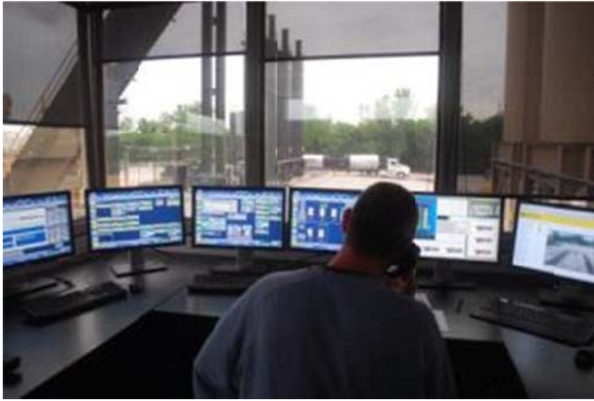
(a) Control room
