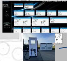
Energy Management System
